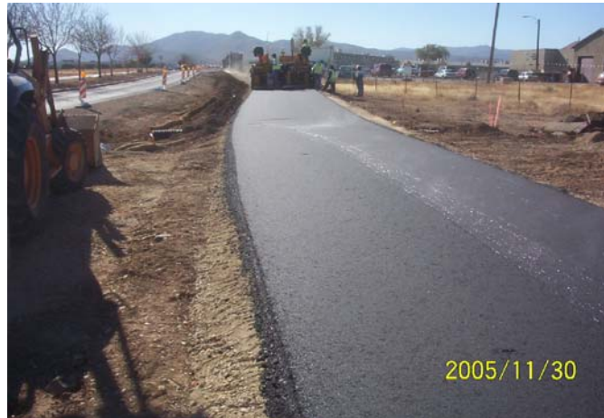
Central Core Path (Phase I) in progress. Lake Valley Road facing south, Liberty Elementary School on the right.
